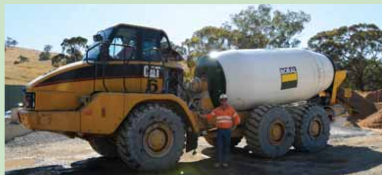
Boral Project Manager Damien Smyth stands by one of the new award-winning agi trucks, which have been purpose built for underground conditions (driver Gerry Juffermans).
