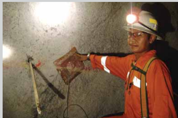
Geotechnical Engineer Asep Wahyudin checks one of the 'black' non galvanized rock bolts and plates in Gosowong's underground: the use of which has reduced the cost of support materials by a fifth whilst maintaining safety standards.
